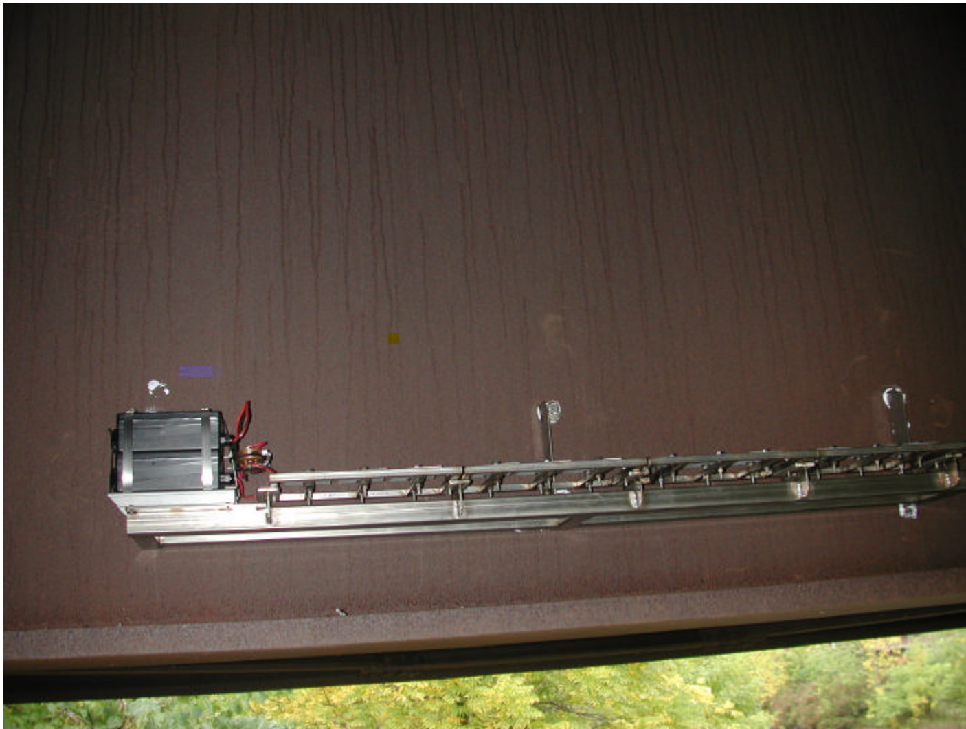
Photograph 19: Specimen Rack 3 installed at location 3MN at East abutment.
