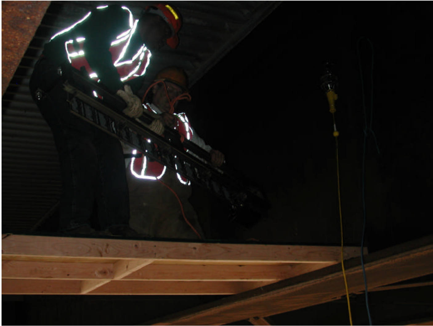
Photograph 14: Specimen Rack 2 being snatched by NYSDOT “skeletons”.
