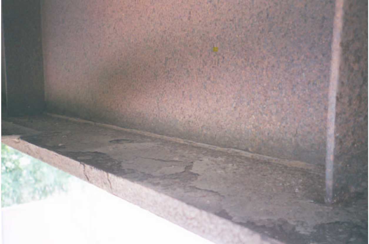
Photograph 2: Moore Drive Bridge, Rochester NY. Corrosion of Girder 4 north web and bottom flange at location 4G (above center lane of I-390 N).
