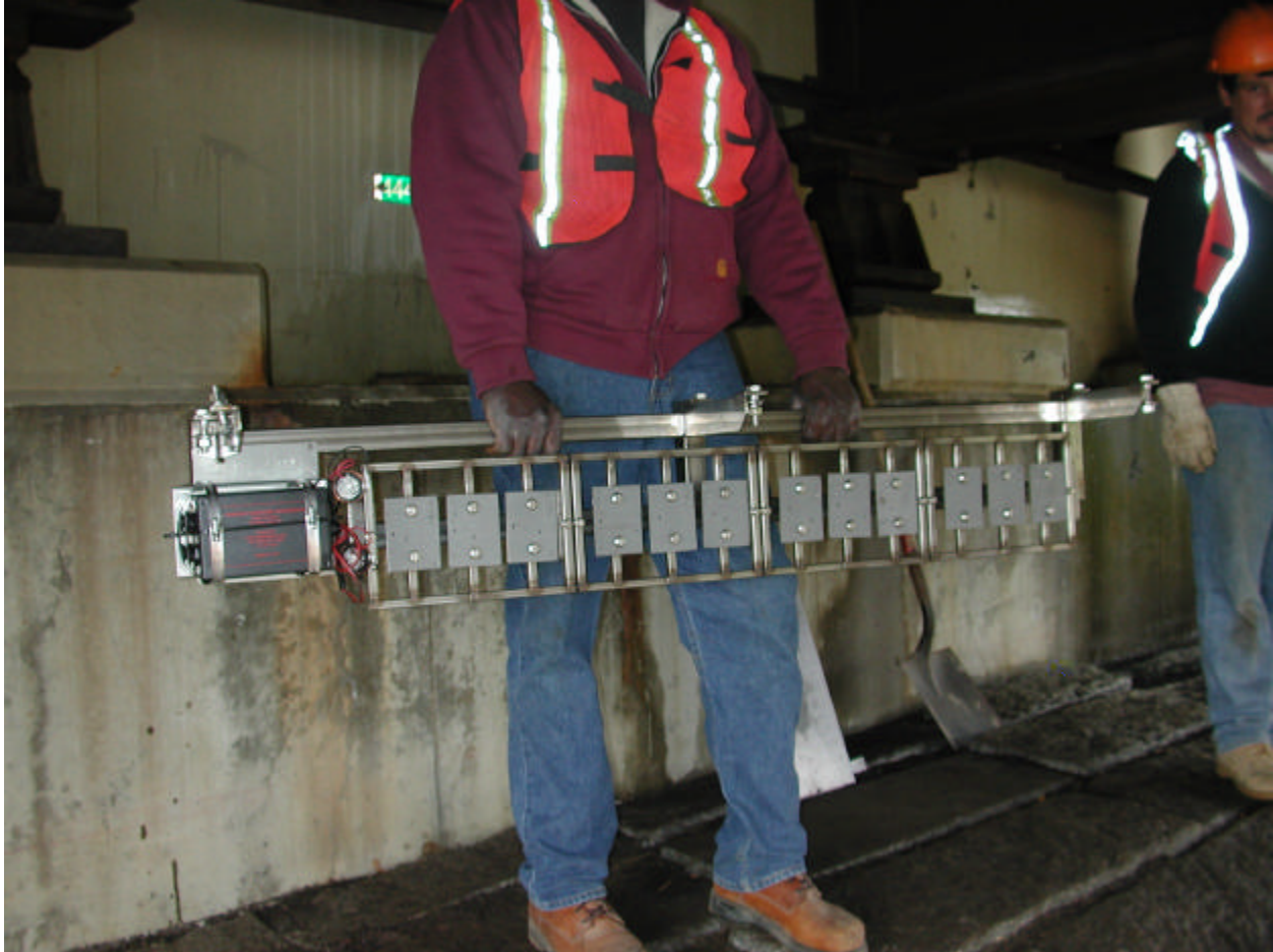
Photograph 12: Specimen Rack 2 ready for installation with Corrosion Monitors attached. Taken at Moore Drive Bridge, West Abutment.
